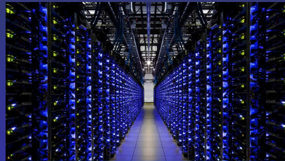
Cooling data centers
